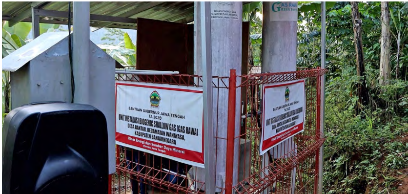
Unit instalasi Biogenic Shallow Gas (BSG) atau gas rawa di Desa Bantar, Kec. Wanayasa, Banjarnegara, Jawa Tengah.
